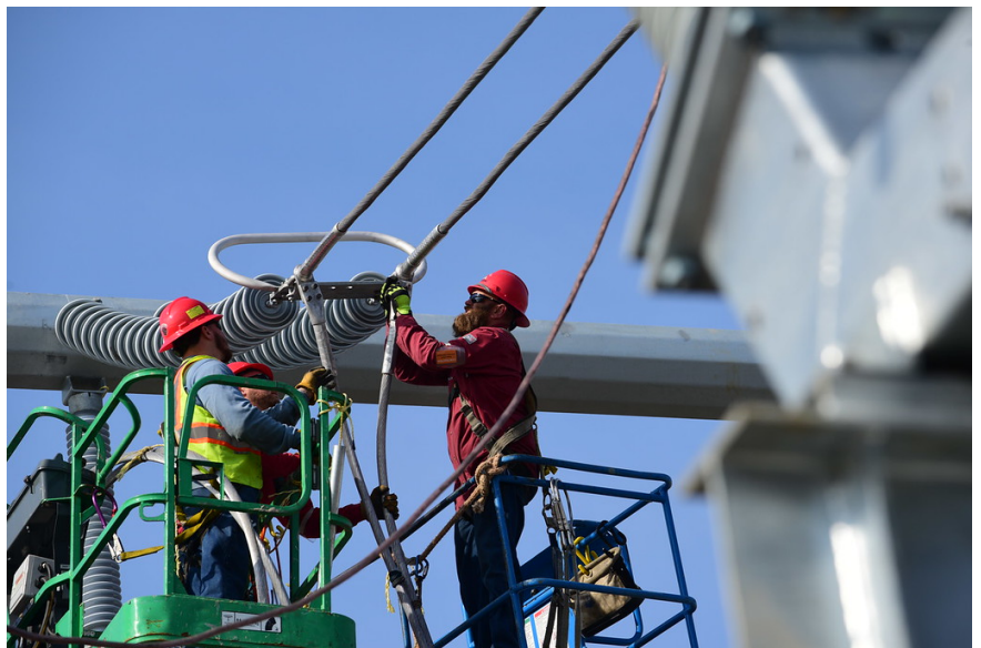
Transmission line workers conduct efforts to safely construct the work near the Goethals Substation in Staten Island, NY
